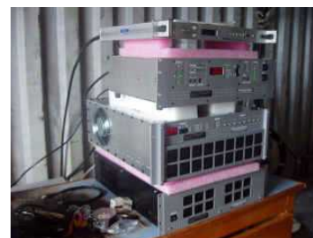
The added transmission power in these equipments
